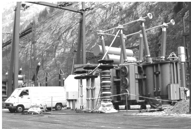
Figure 4 - Off-line test set-up for PD-diagnosis on a 380/220-kV separated regulating transformer unit using a frequency tuned series resonance test set. The resonance reactors and capacitors are situated in the center of the photograph.
