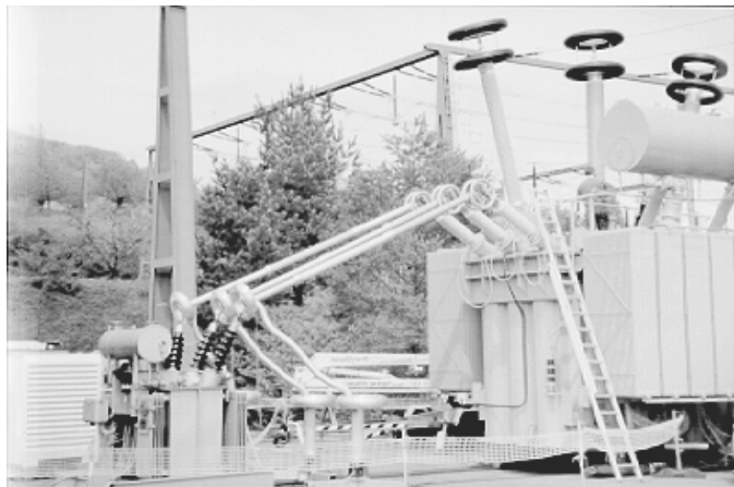
Figure 2 - Off-line test set-up for PD-diagnosis on a 220/50-kV transformer using a 300 kVA diesel generator unit and a step-up transformer 0.4/50 kV (left). Transformer under test with torus electrodes at the HV-bushings to avoid corona discharges (right).
